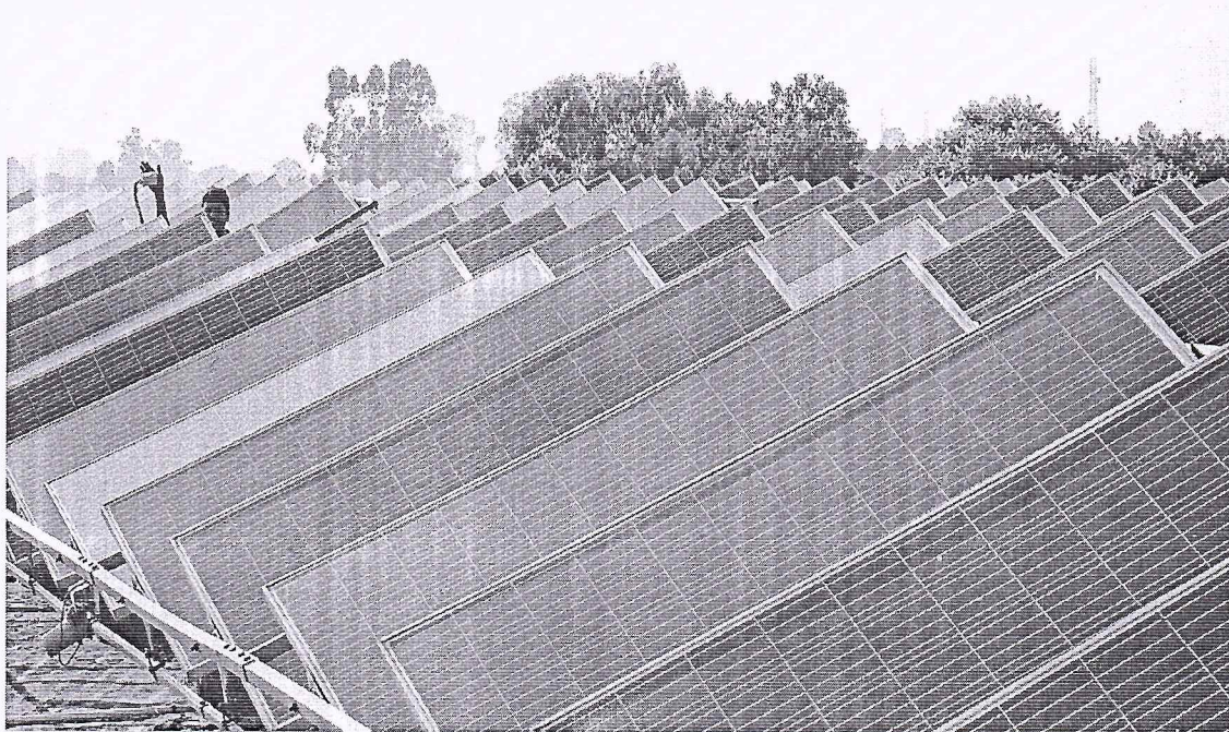
Installed Roof-Top Solar Panel
